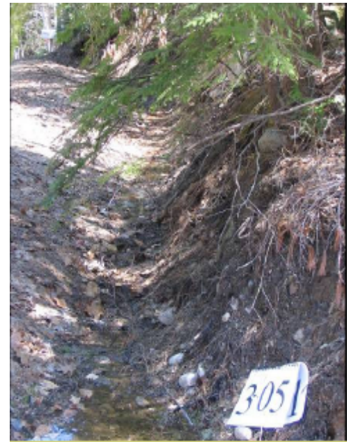
Private road erosion site
